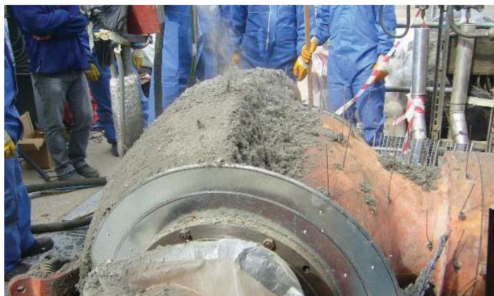
Fire protection in turbine construction at Warsaw University of Technology
